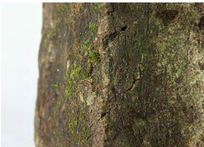
Image 04 : Live mosses The new flood-resilient interior - comprising drainage barriers, closed cell insulation and plywood cladding - allows the existing brick superstructure to be home to free-growing microbes.
